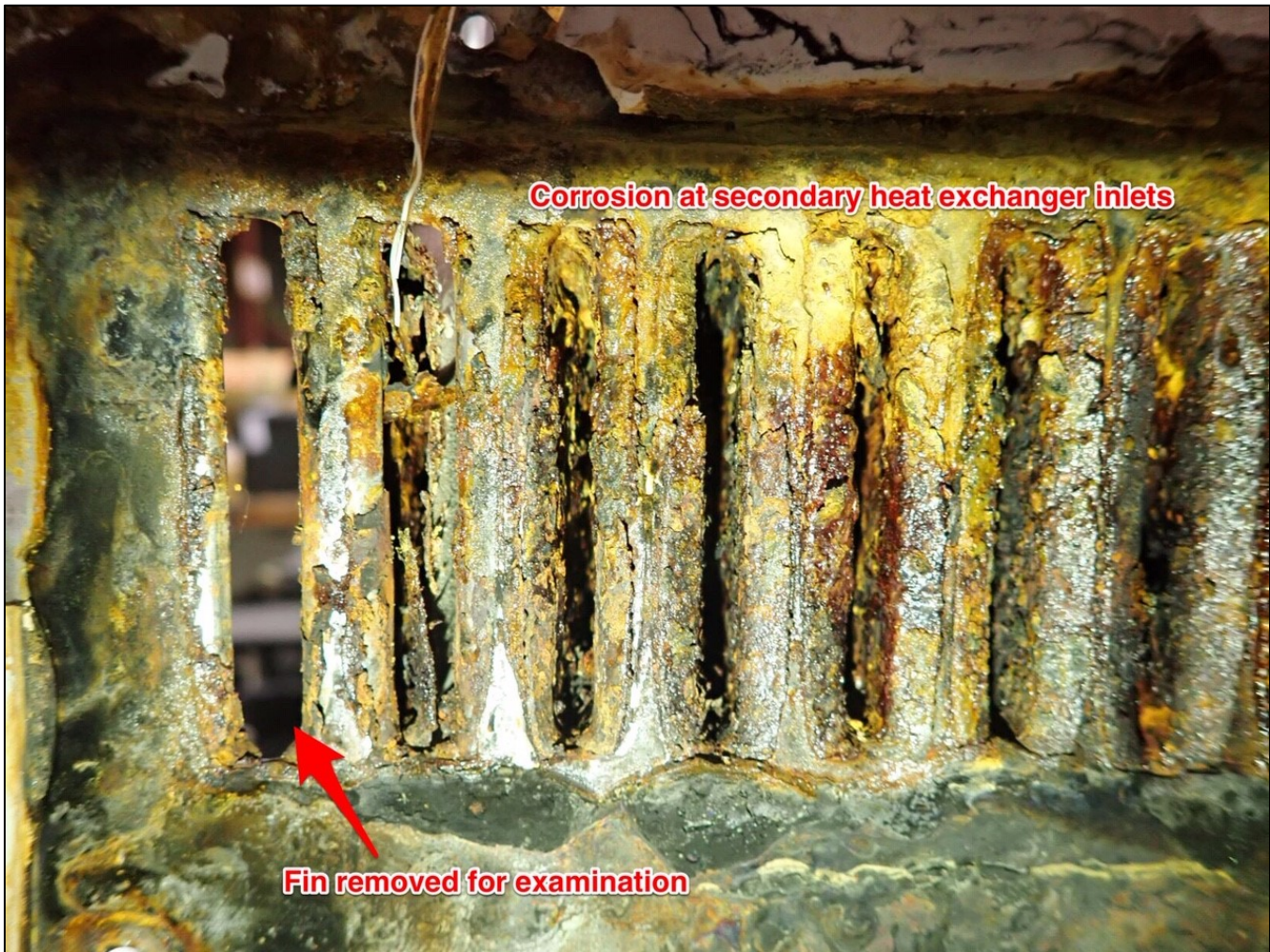
Image 11 – Secondary heat exchanger tube inlets with one tube completely removed for examination. Image shows corrosion, delamination of polypropylene liner and restricted passages.
