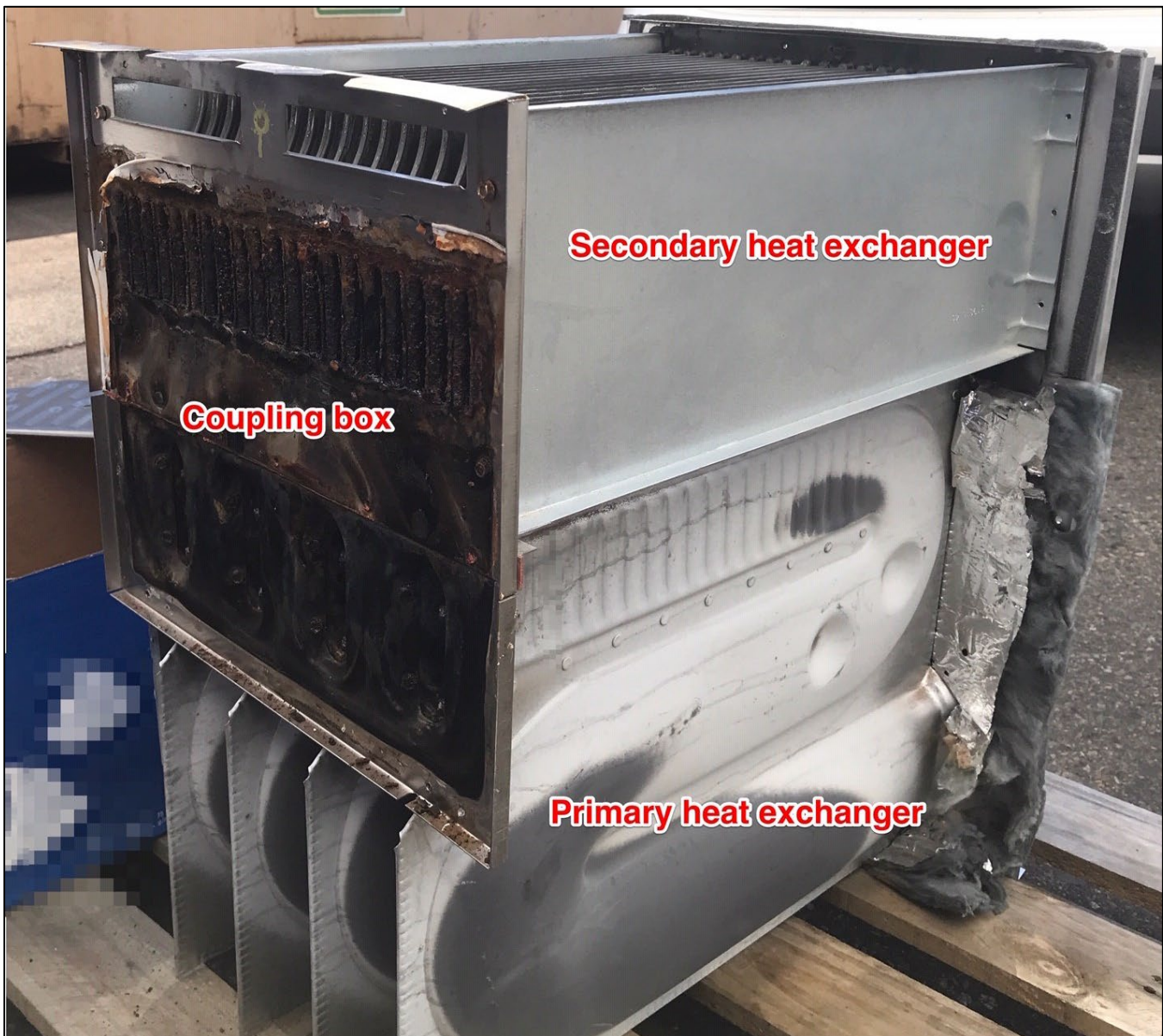
Image 8 – Complete heat exchanger assembly removed from furnace for examination (coupling box cover and baffle removed in this image). The heat exchanger is sitting upside down from its up flow operational position. Combustion products from the gas burners travel through the S-shaped primary heat exchanger to the coupling box and then pass through the secondary heat exchanger tubes before being expelled to the outdoors by the draft inducer fan through the vent piping.
