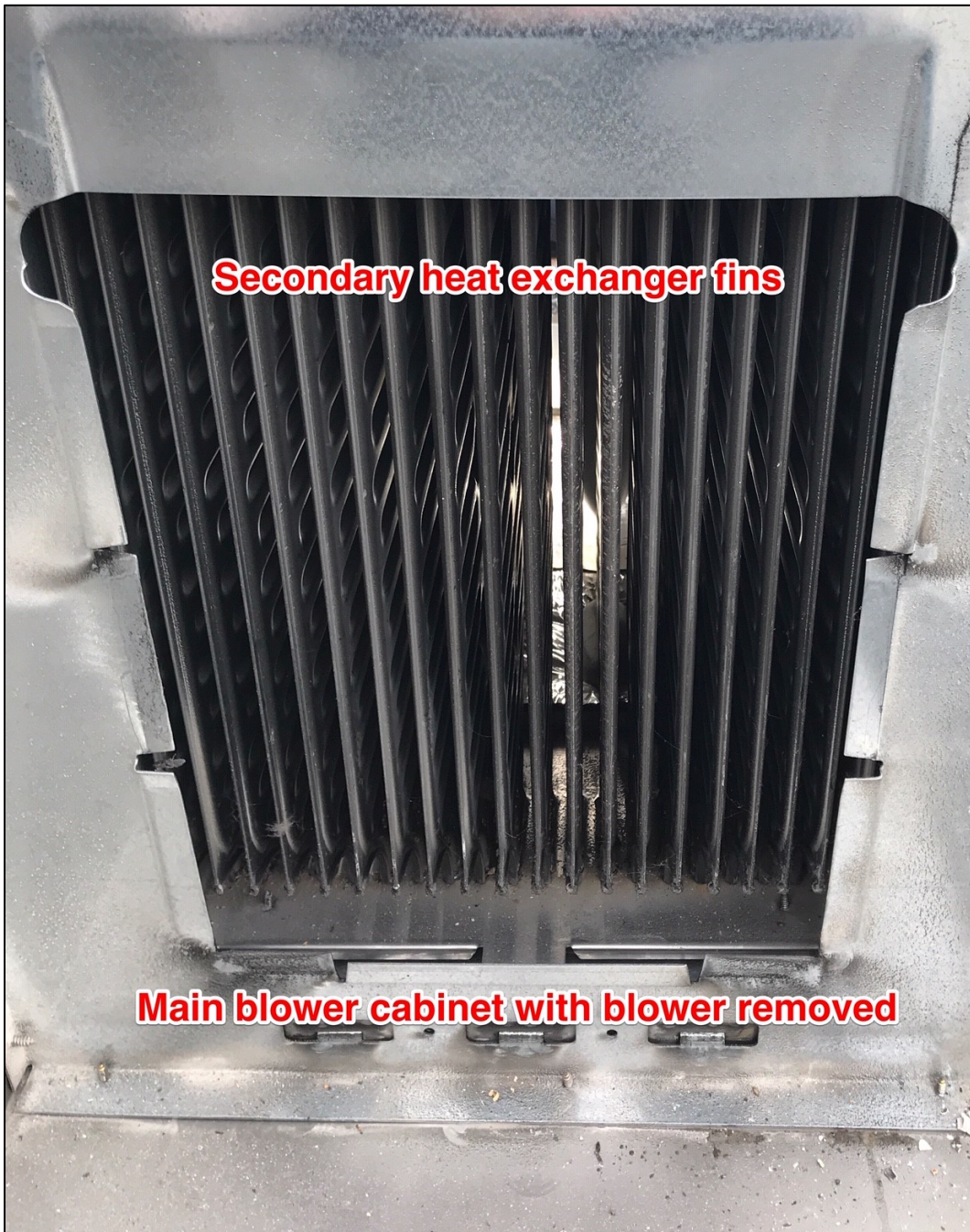
Image 7 - The main blower blows air up through the secondary heat exchanger then through the primary heat exchanger above it.
