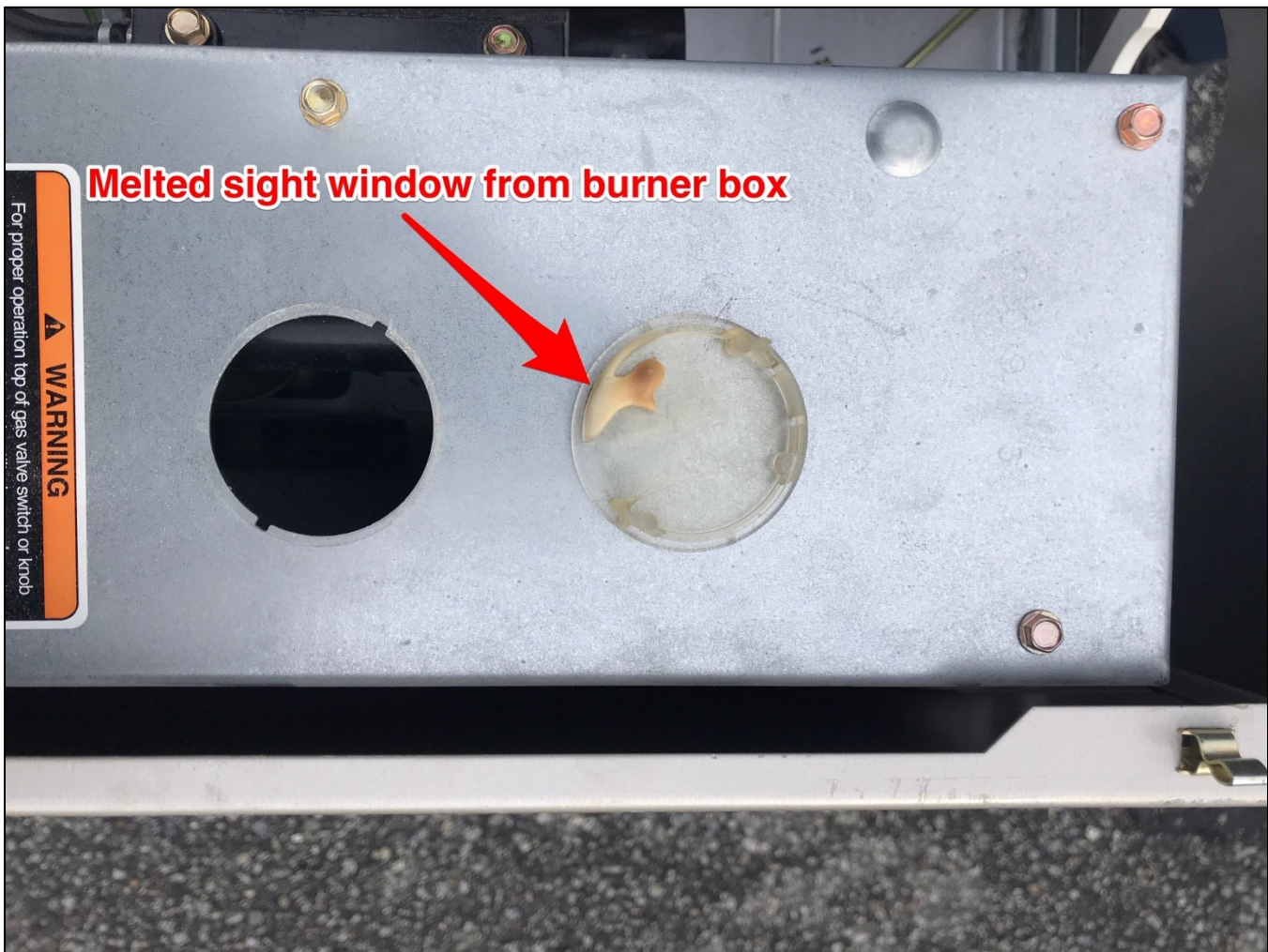
Image 4 - Plastic sight window removed from burner box showing signs of melting from insufficient air flow and flame rollout.
