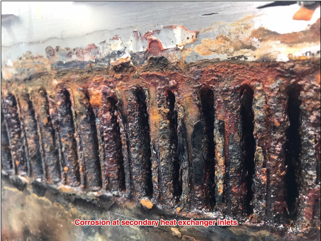
Image 9 – Close up of secondary heat exchanger tube inlets in coupling box showing severe corrosion.
